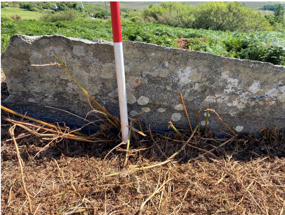
Plate 6 Detail of lichen growth on straight face of cap stone
